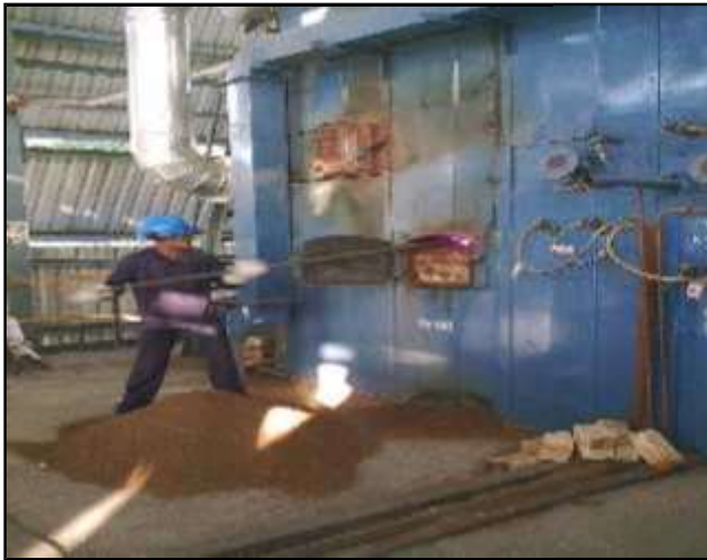
The Fireman Is Checking the Bed & Charging Bed material In Furnace of F.B.C Boiler.
