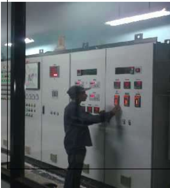
The Boiler Operator Is Operating the Digital Control Panel Of the Boiler
