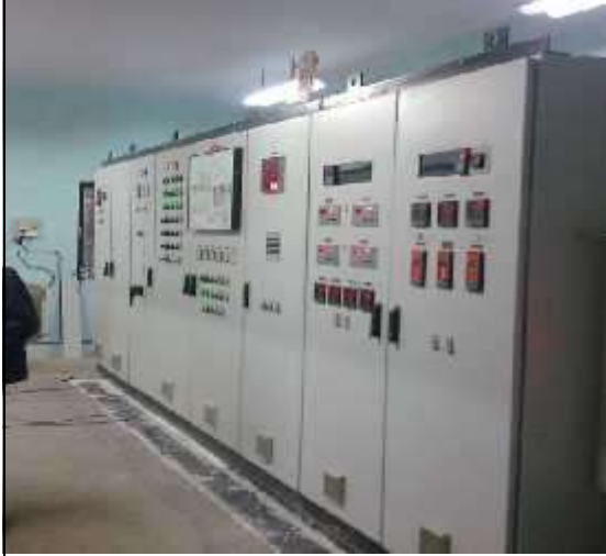
Panel Board of the Boiler with Pneumatic Control
