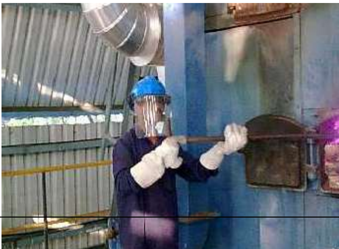
The Fireman Is Checking the Bed & Charging the Bed material In Furnace of F.B.C Boiler
